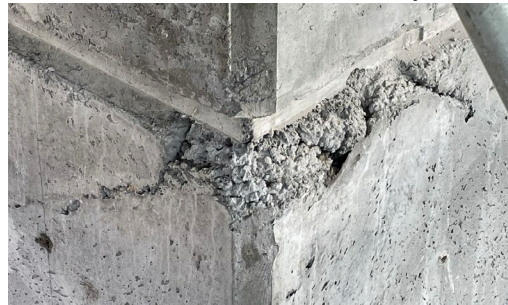
Figure 2 Honeycombing present on Pier D4 from T2021-Q
